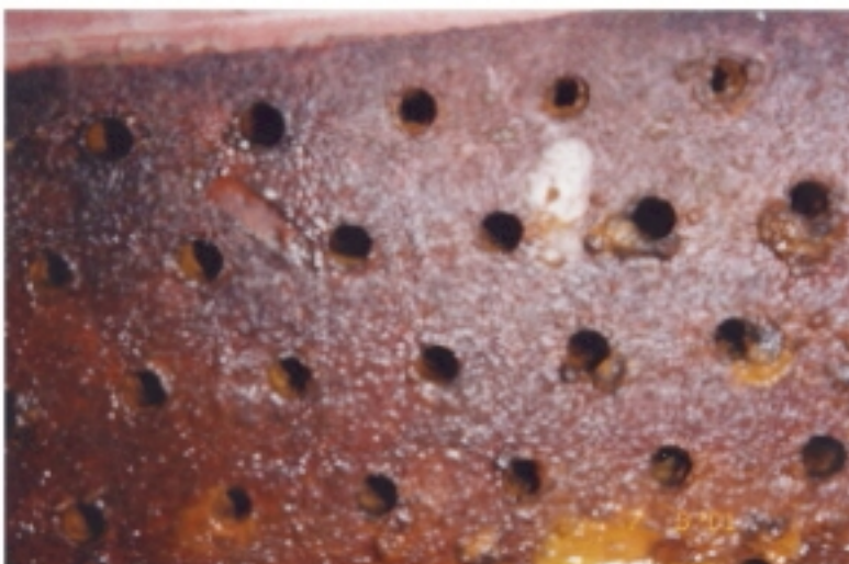
Four months after installation. Muddy scale, soft and easily removed
